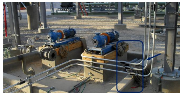
Figure 3. Electrical raceways (3) with TB outlet bodies and drain fittings.
