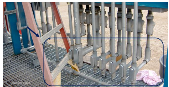
Figure 4. Electrical raceways with TB outlet bodies and drain fittings, at low points in the raceways.
