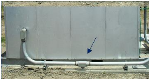
Figure 1. Electrical raceway installation, with T body outlet and drain fitting, installed at low point of raceway.
